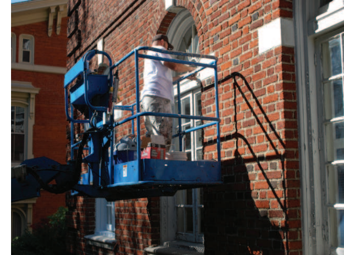
Painting crews scrape old paint and apply coats of fresh paint to the window frames of the Orange Street side of YW's building. The window painting is part of HUD requirements for Section 8 housing.
